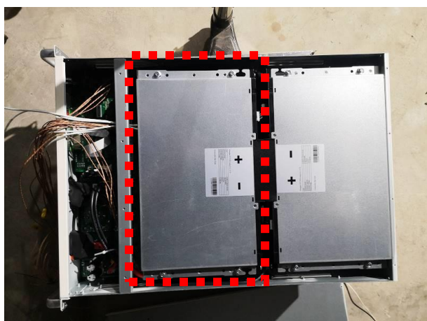
Figure 5c. Internal view 03 of battery module.
