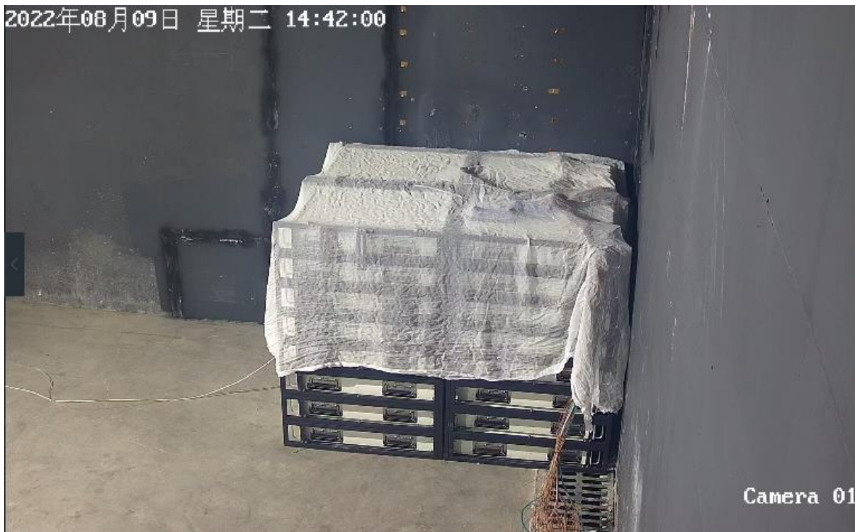
Figure 12. Photo 01 of initiating BESS unit and target BESS units during test.
