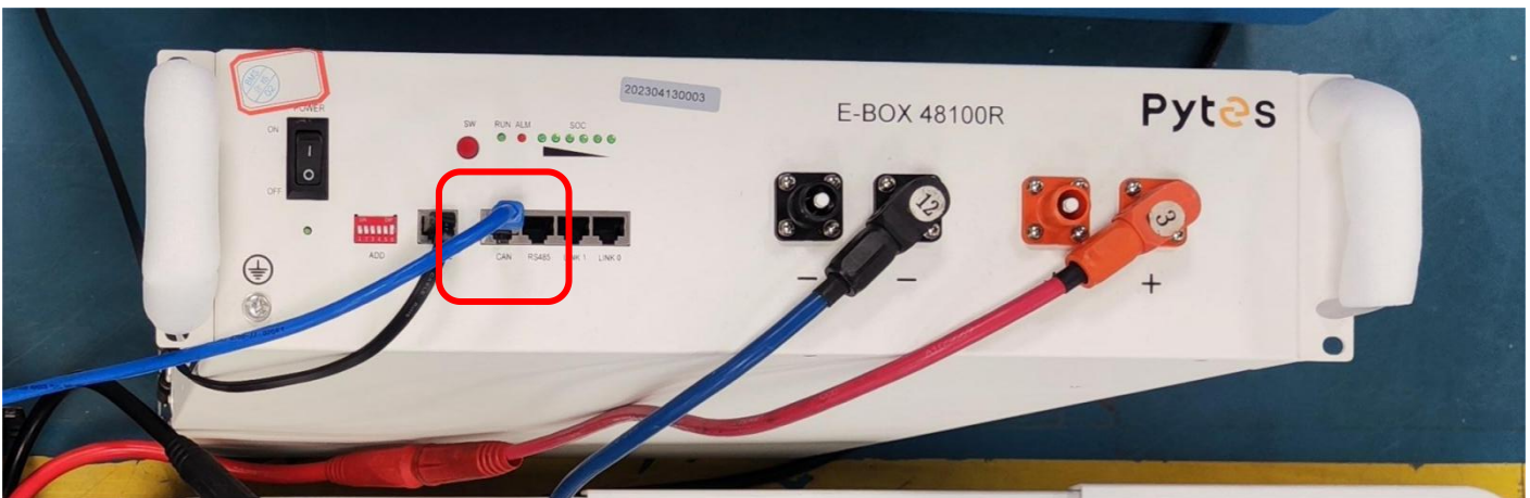
Figure 1.1.3 battery comm and power cable connection
